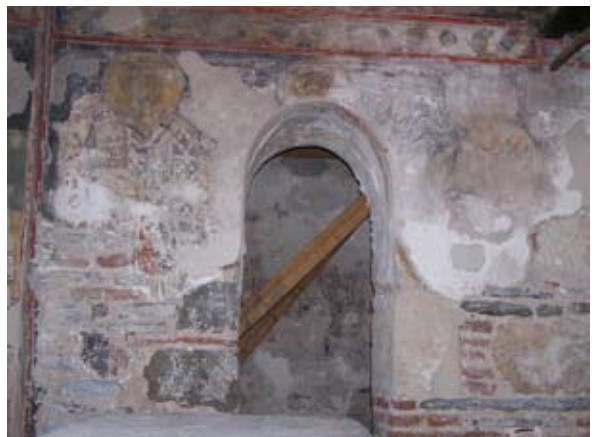
Fig. 15. Current problems – walls
