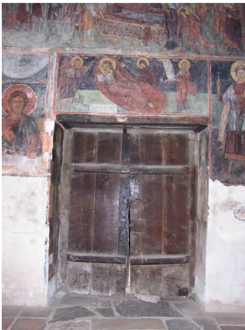
Fig. 16. Current problems – openings
