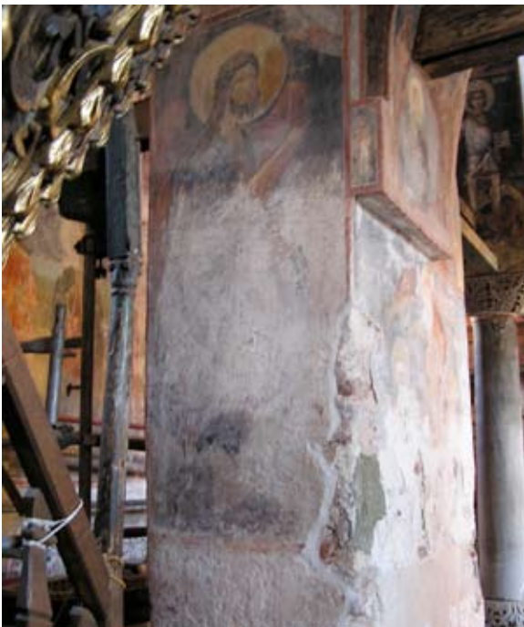
Fig. 14. Current problems – walls
